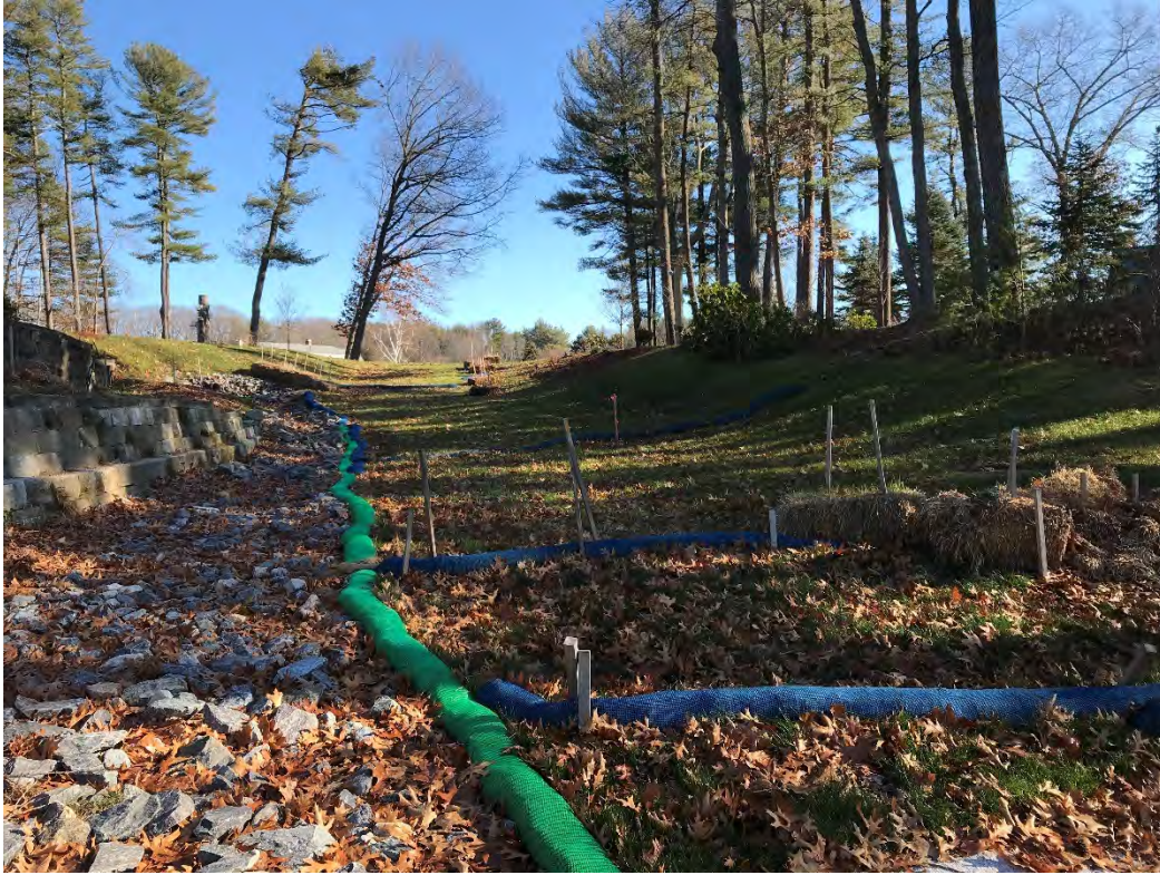
Fig 5: Slope above the manhole at Gundalow Landing/east side of the bay. Viewing east. (12-15-20)
