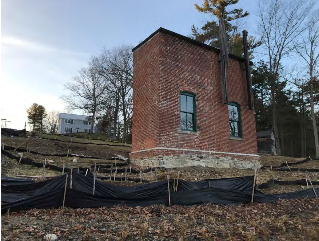
Fig 3: Cable house post-restoration and scaffolding removal at the Eversource property/west side of the bay. Viewing northwest. (12-11-20)
